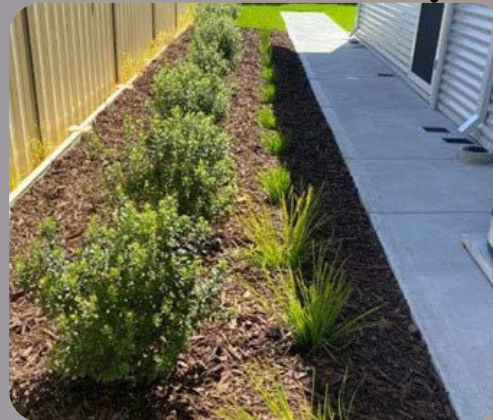
Figure 125. 1m concrete apron installed to perimeter of dwelling and graded toward garden beds. Low maintenance species planted at required 2 plants/m 2 .
