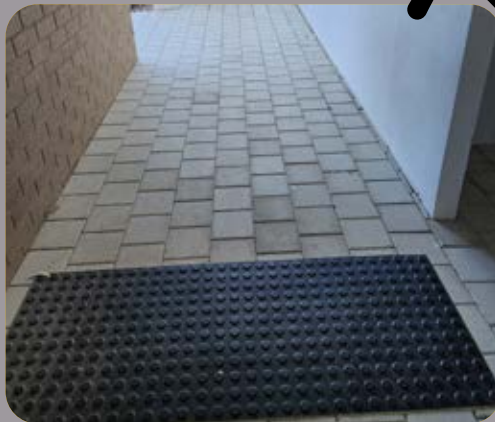
Figure 90. Stick on TGSi's are not sufficiently robust. TGSIs only required where ramps or stairs are needed.
