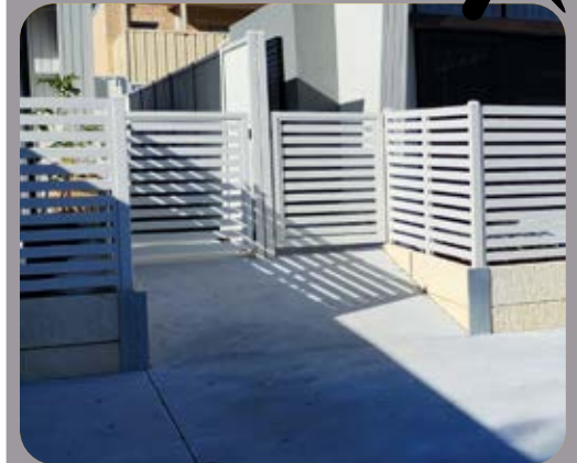
Figure 88. Primary entries to dwellings are steep with non-conforming ramps, no handrails, kickguards or TGSIs
