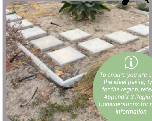
Figure 22. Height of gap between pavers is a trip hazard. Space needs to be filled in with material to maintain flush edge.
