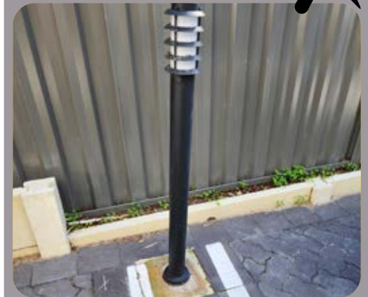
Figure 80. Communal space lighting can be damaged and vandalised.
