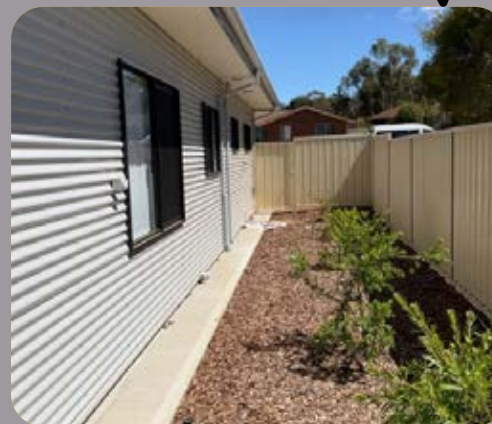
Figure 117. Concrete apron installed. Small shrubs installed to minimise conflict with fence or dwelling.
