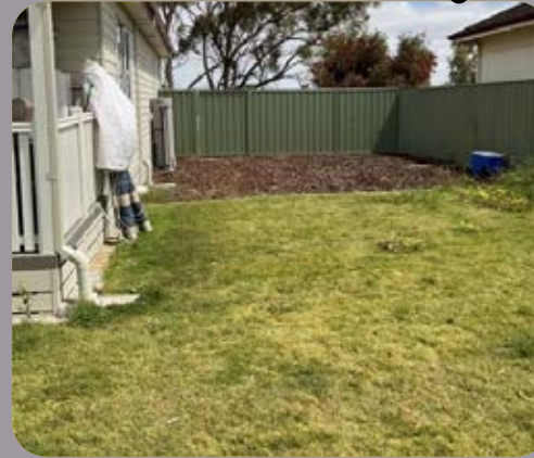
Figure 116. An excessive use of turf. No concrete apron installed to property.
