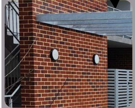
Figure 79. Communal space lighting is integrated into built form.
