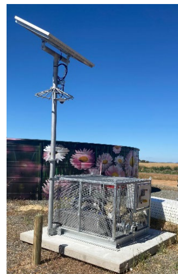
Tank, electric swipe card and pump for bore
