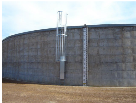
Goodland's Tank and gauge
