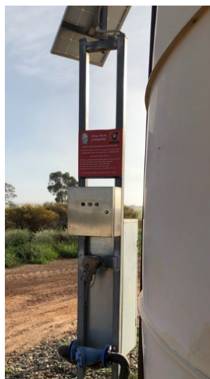
Swipe card standpipe system
