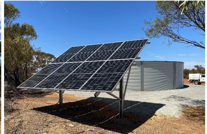
Solar array and pump
