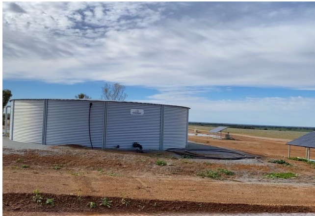
Solar array adjacent to tanks
