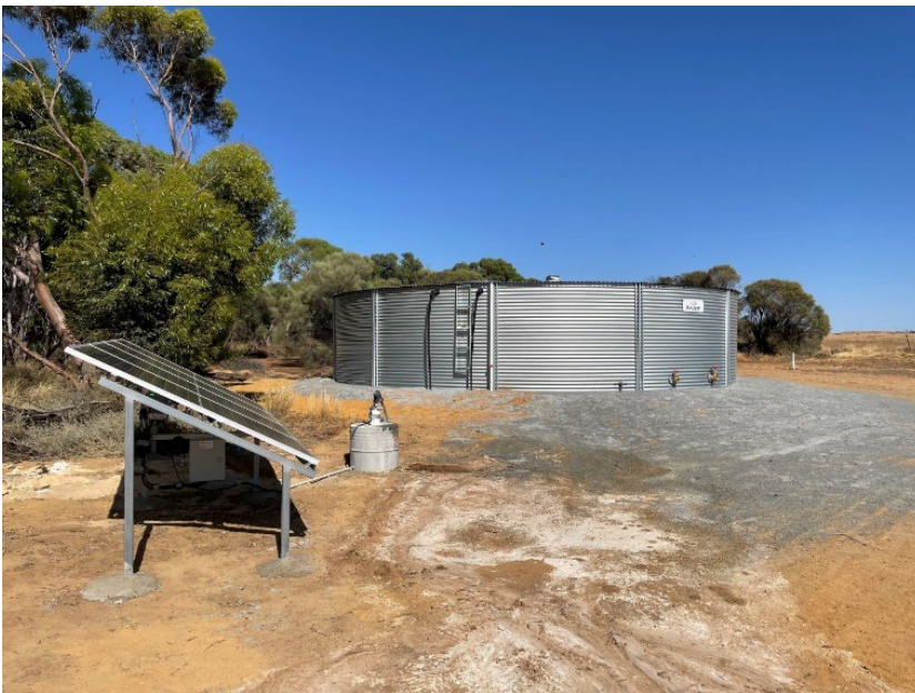
Solar array and pump
