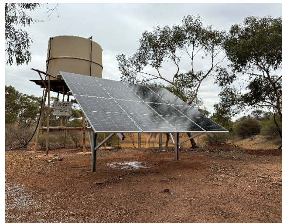
Solar array and pump (2024)
