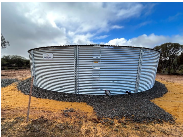
Morawa Yalgoo Road tank
