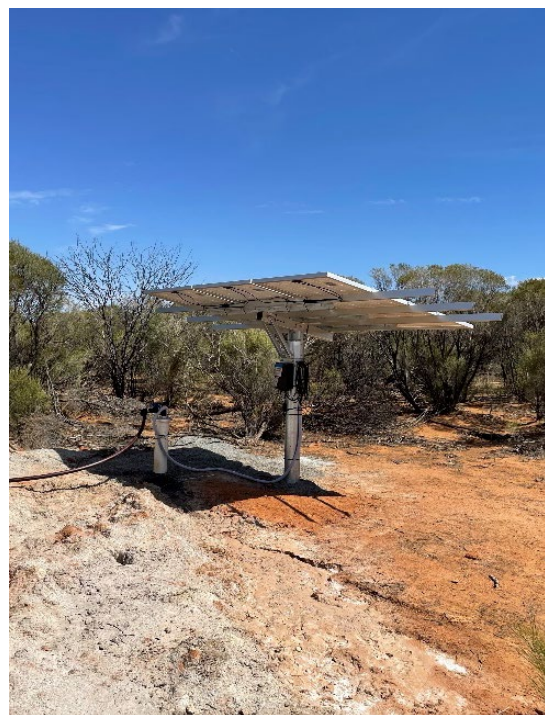
Solar panels and pump
