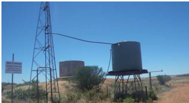
Tank, windmill and standpipe
