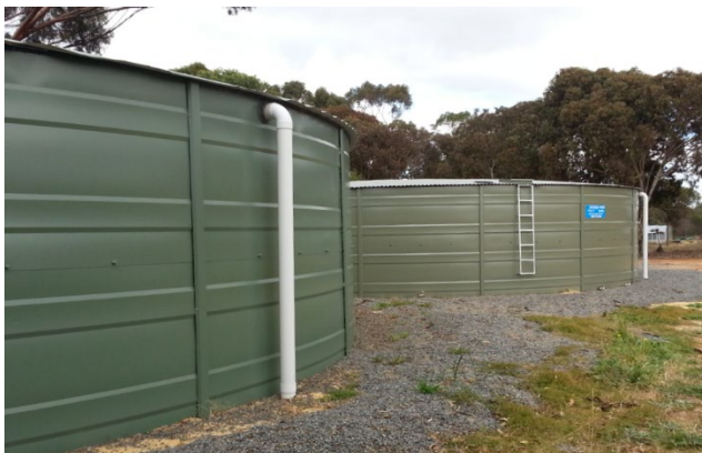
Tanks located at Leisure Centre filled with Water Corporation reclaimed water
