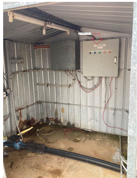
Pump shed controller
