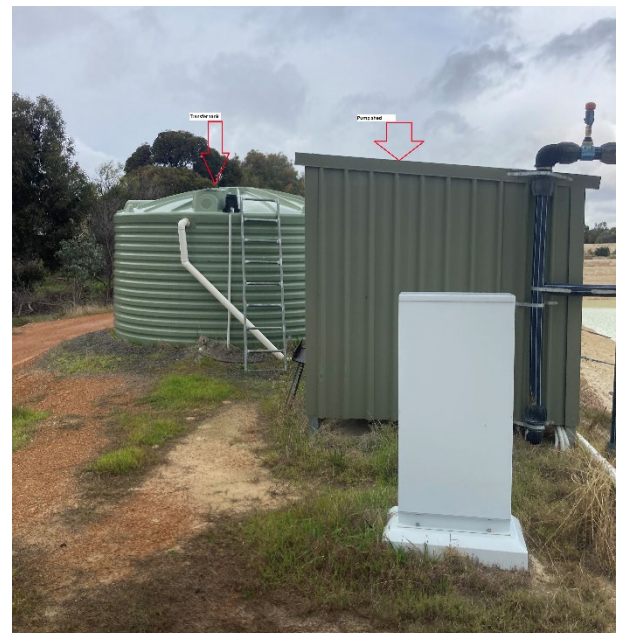
Pump shed and transfer tank
