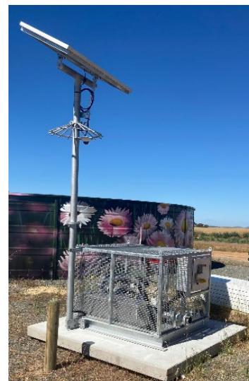
Tank, electric swipe card and pump for bore
