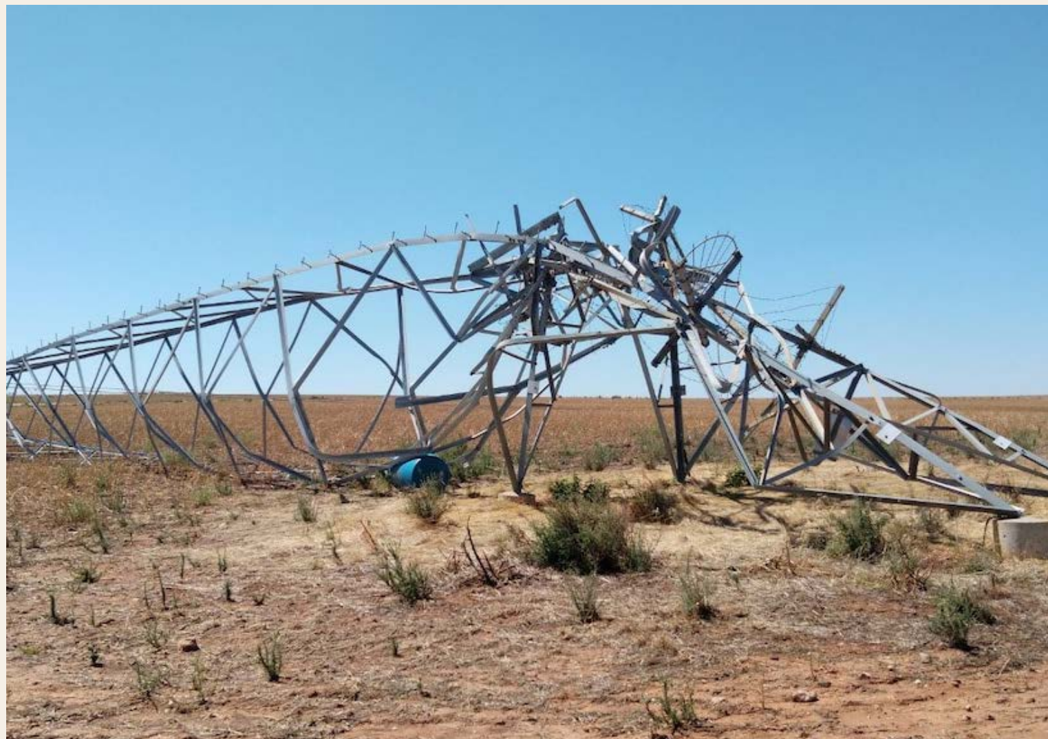
Collapsed Transmission tower on the Kondinin to Merredin line Source: Western Power
