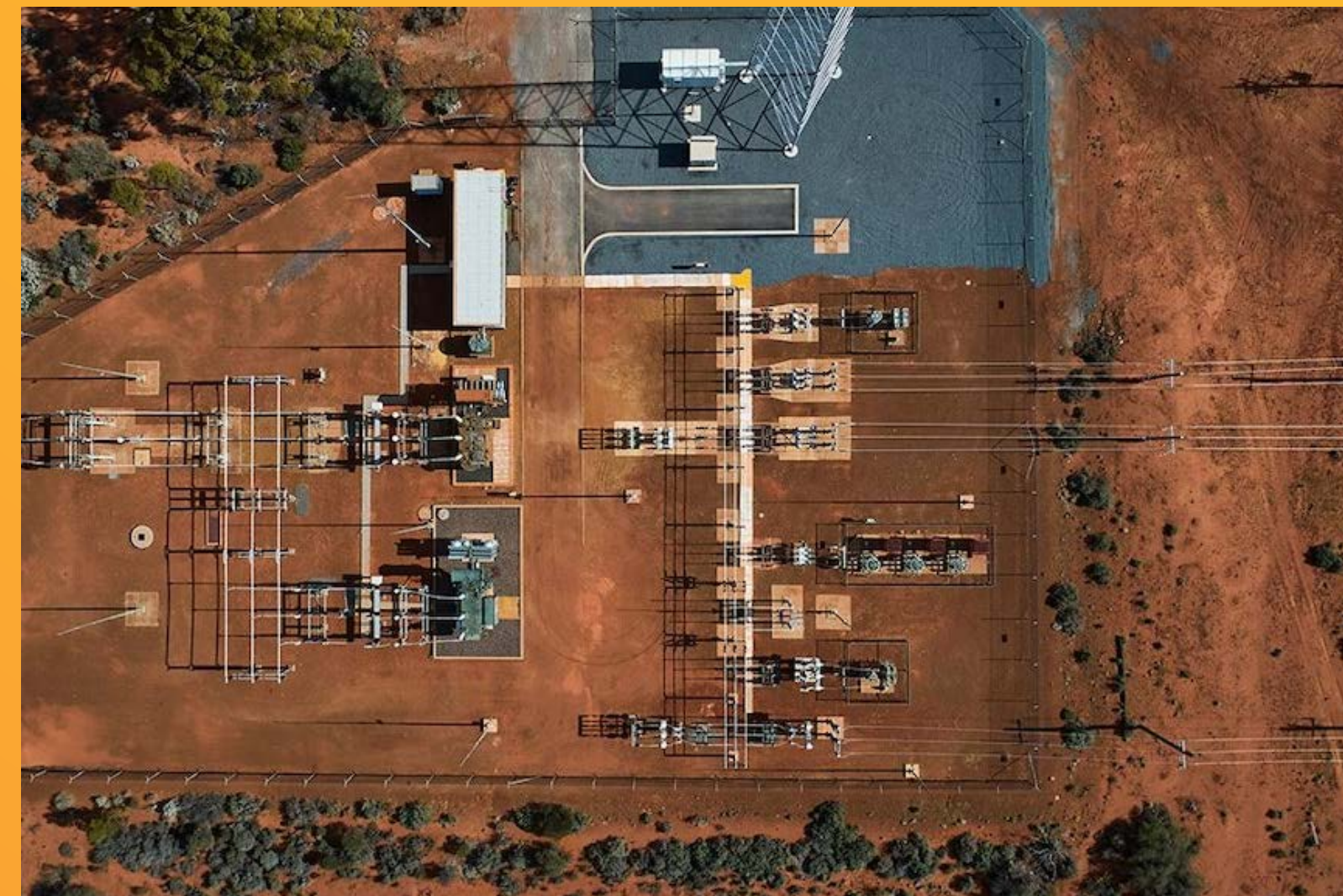
Aerial view of Western Power's sub-station in West Kalgoorlie Source: Western Power
