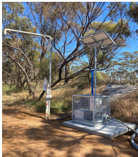
Standpipe at located on Garnett Road pull-through
