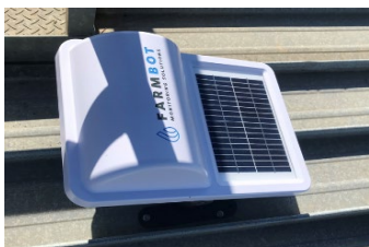
Farm bot positioned on top of tank
