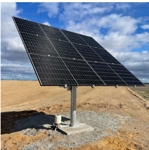
Solar array and pump
