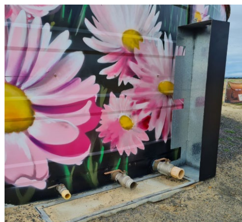
Coupling on southern tank
