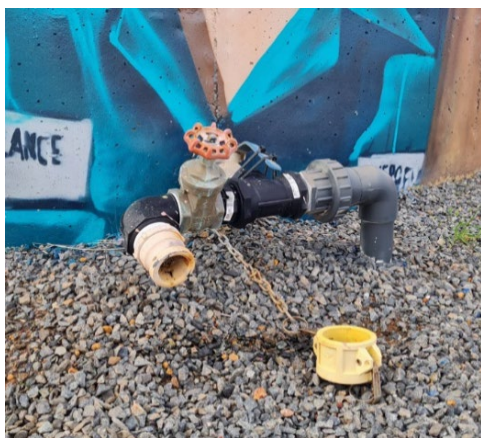
Coupling on northern tank
