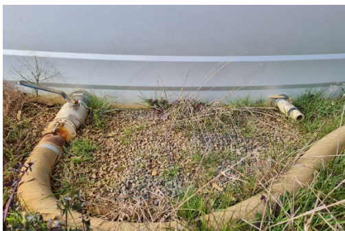
Fill point on steel tank 2 x 50, 80 and 100 mm
