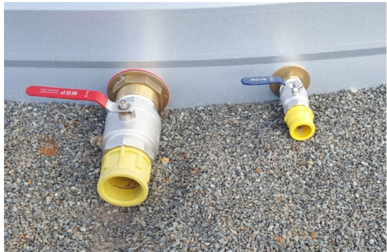
Couplings on tank
