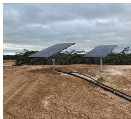
Solar pump on dam
