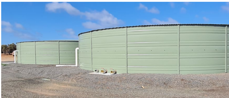
Tanks and camlock outlets
