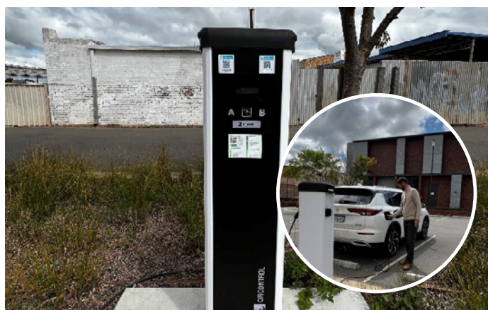
Images of charger and person EV charging at the Shire of Katanning Council Building. Images supplied by the Shire of Katanning in September 2024.
