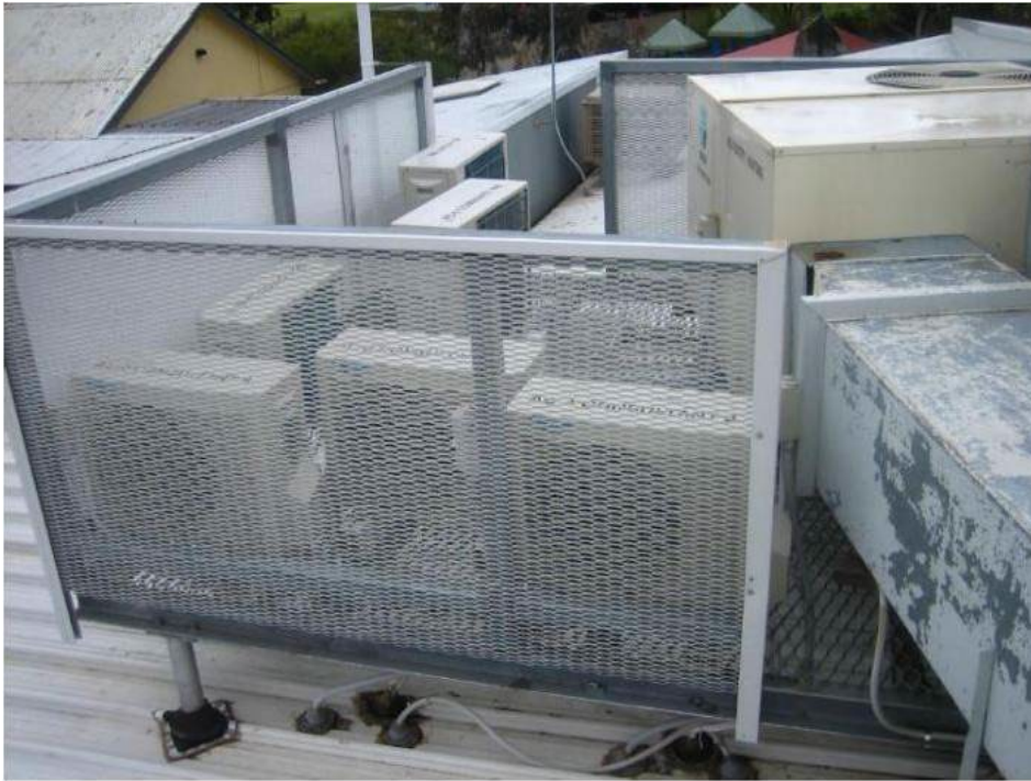
Figure 8: Example of poorly accessible mechanical equipment
