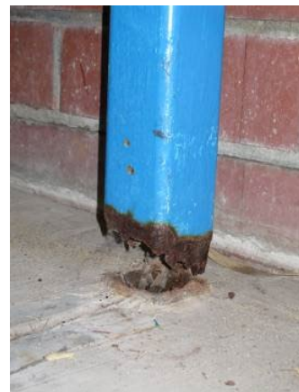
Figure 7: Potential effects of poor corrosion protection.
