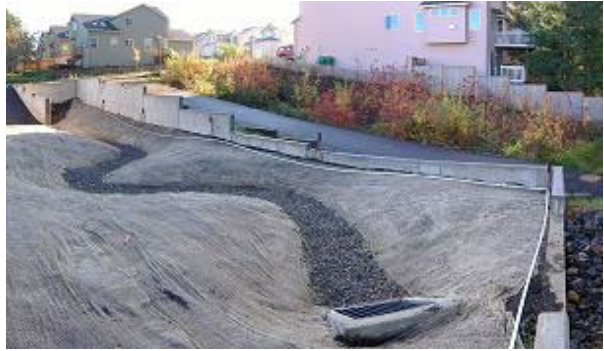
Figure 2: Two bio-swales for a housing development. The one in the foreground is under construction, while the one in the background is already established.
