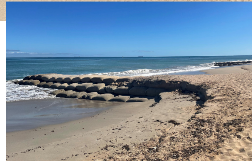
Stage 2 of the Sunset Beach stabilisation project using Geosynthetic Sand Containers (GSC) and sand nourishment. Photos by DoT.
