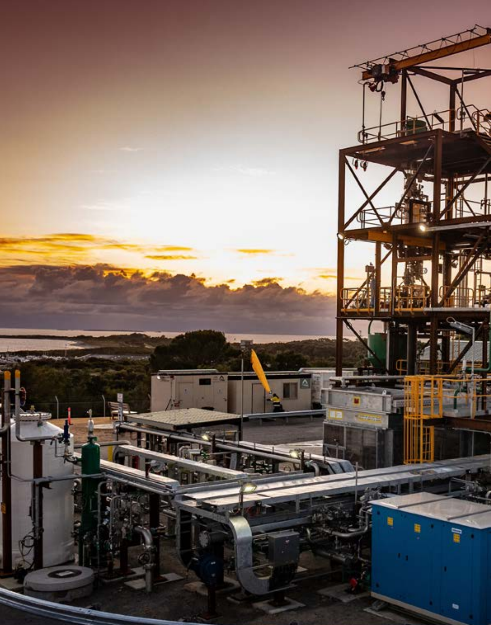
Hazer Commercial Demonstration Plant, Perth, Western Australia. CREDIT: Hazer Group Limited © 2022 – All Rights Reserved
