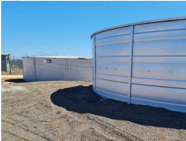
Tank 2 x 250 kL located at sportsgrounds
