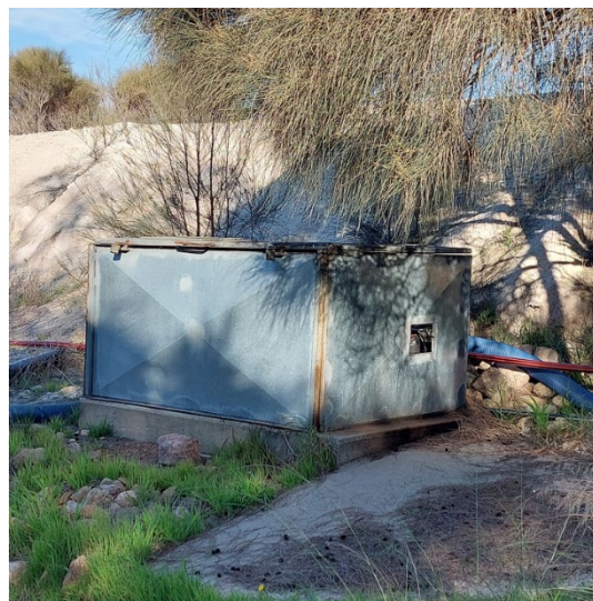
Pump at standpipe
