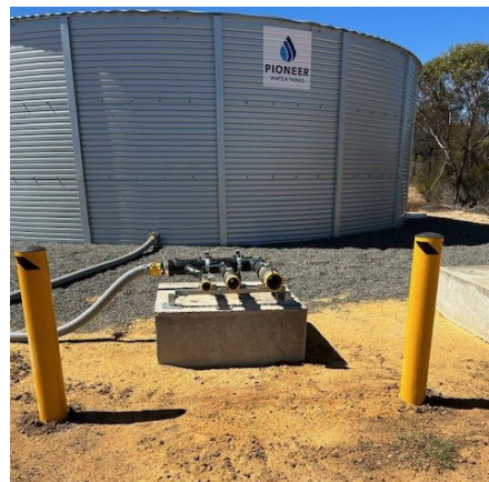
Manifold outlet set-up
