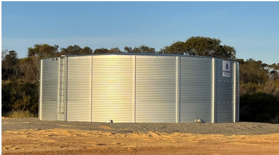
291 kL tank installed in 2023
