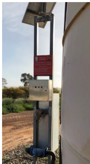
Swipe card standpipe system
