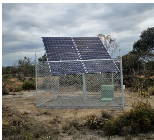
Bore with solar pump
