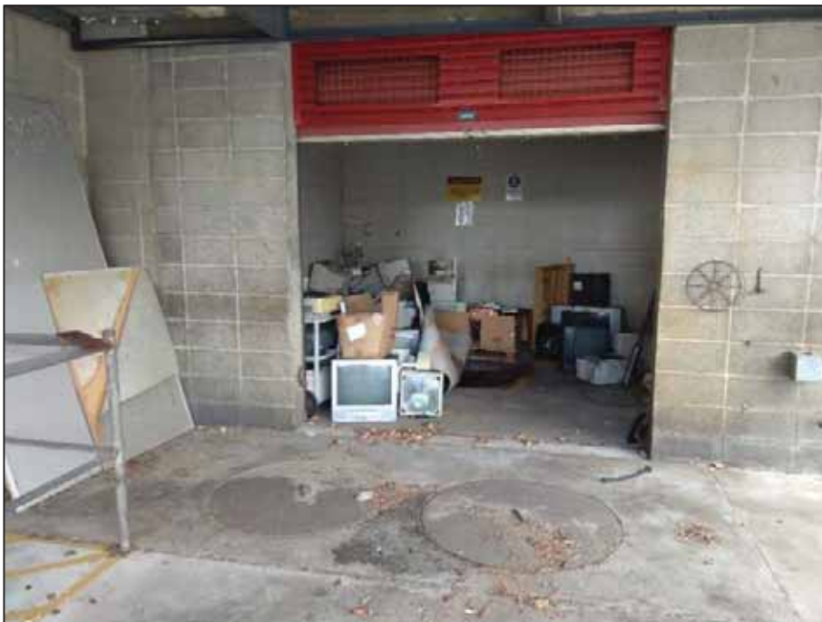
Plate 2: TIT present outside a possible wash bay on the east side of Building J with a drain visible within the centre of the room.
