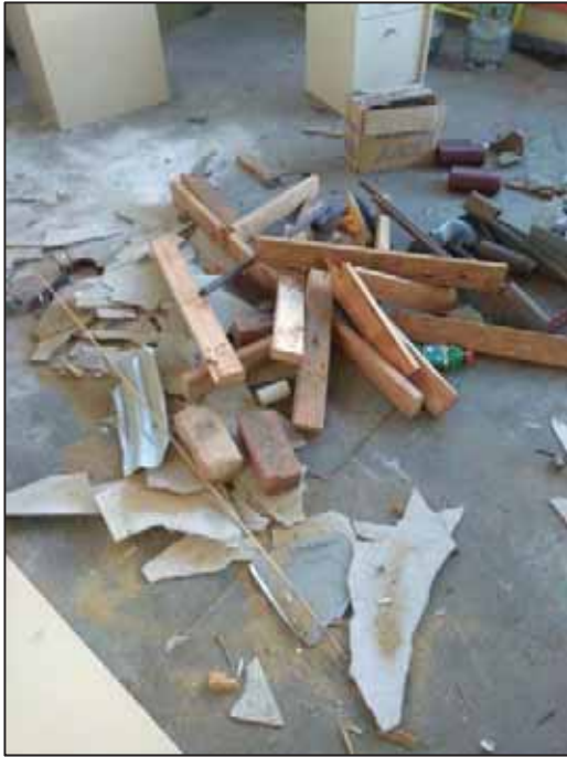
Plate 5: Broken FCM pieces lying on the ground within Building M.
