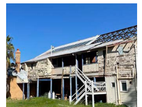
Figure 4: A Dilapidated Home in Bencubbin
