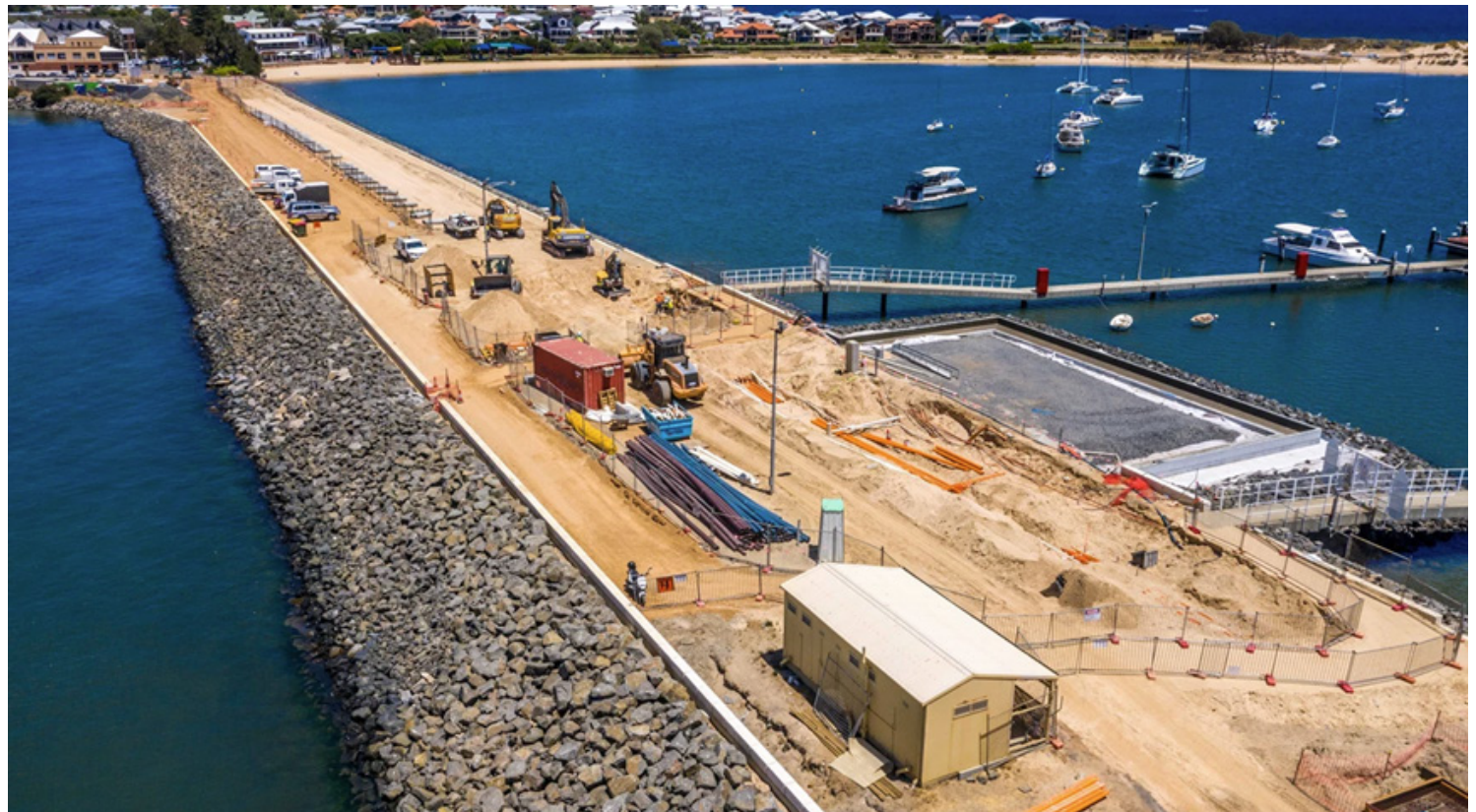
Works at the Transforming Bunbury's Waterfront project; laying of foundations for a multi-purpose building on the Jetty Road causeway x
