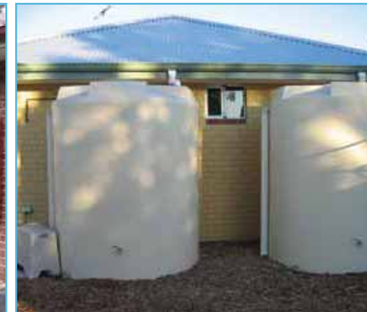
Poly domestic rainwater tanks
