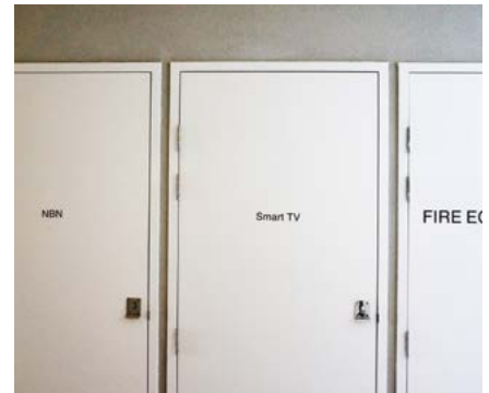
Photo 4.18b This apartment is fibre-to-premises ready.
