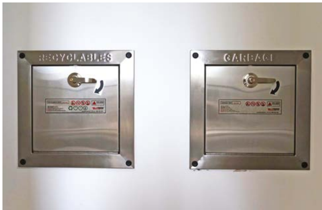
Photo 4.17a Dedicated recycling and waste disposal chutes allow source separation and recycling.
