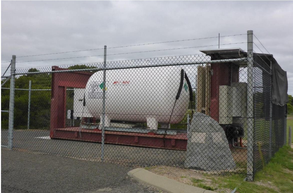
Figure 1 The land-based plant on the eastern side of the Vasse estuary surge barrier
