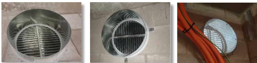
Figure 7: Examples of fire dampers required to protect penetrations through a fire rated wall. (Drost, 2019)
