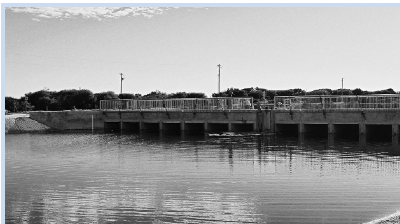
Floodgates on the Vasse Estuary replaced in 2004
