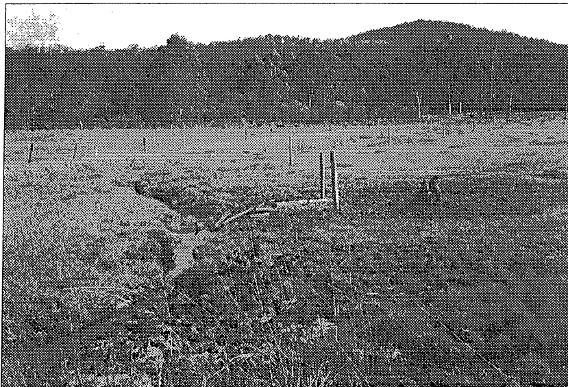
Fencing in progress on a small tributary of the Little River, close to Ocean Beach Road. In this case, the fence ought to be sited further away from the watercourse, in order to allow for several rows of trees and shrubs to be established in the riparian buffer zone.
