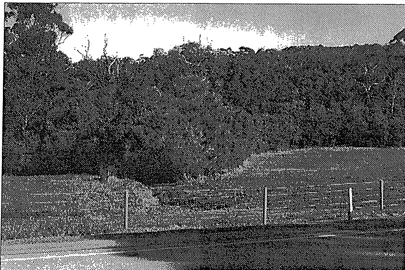
A drain from a culvert off South Coast Highway, in the vicinity of the Lights Road overtaking lane. Such drains need to be stabilised with native revegetation and, where necessary, with riffle and pool zones.
