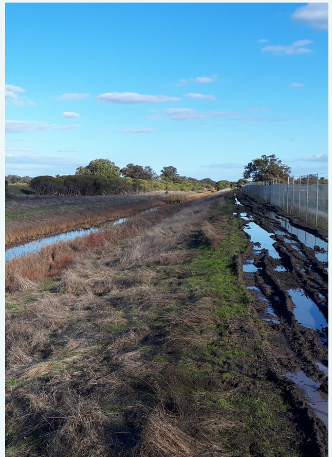
Peel Main Drain, note the waterlogging along the fenceline to the right of the photograph, June 2019.
