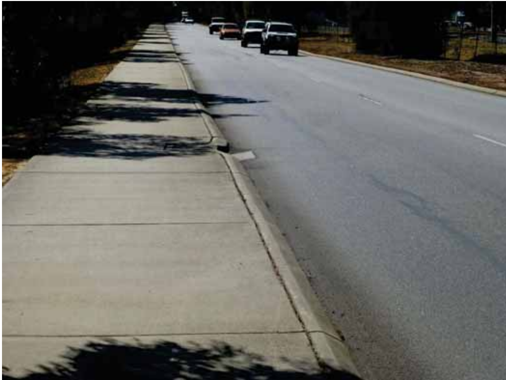
Photograph 5: Surface deflections on Railway Avenue
