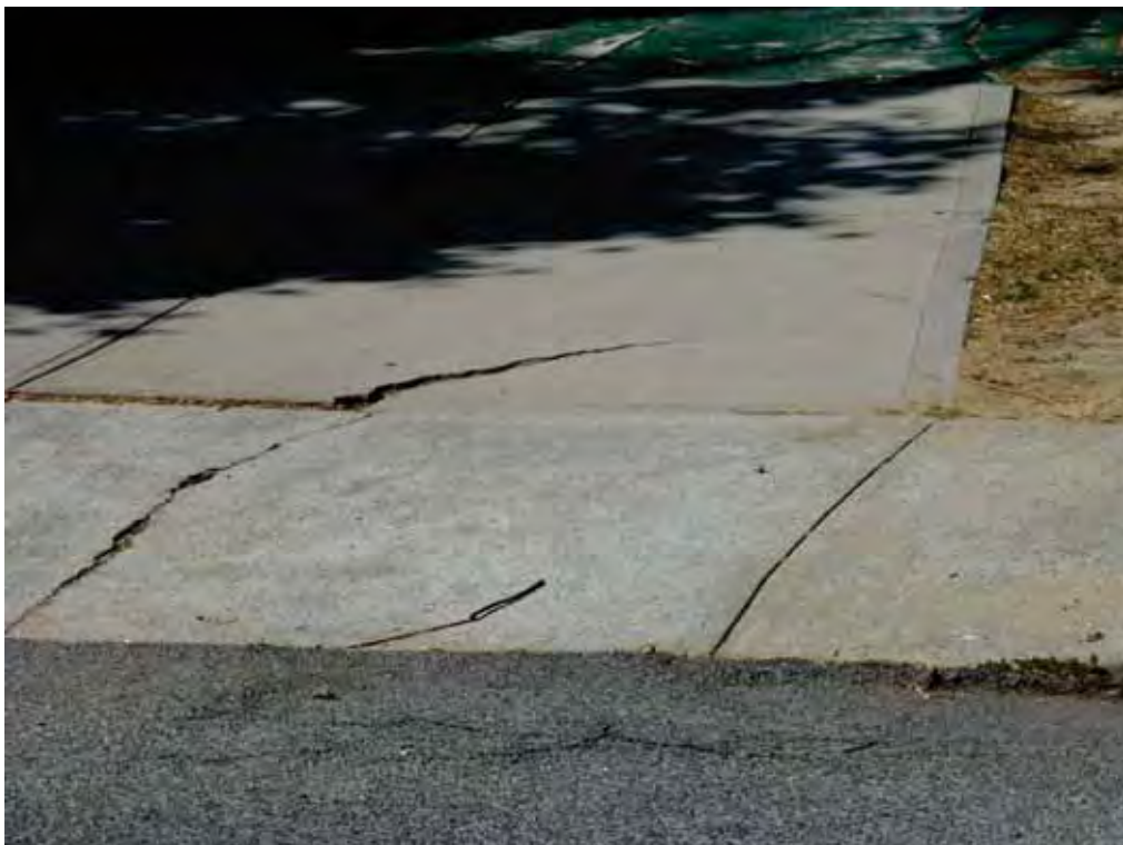
Photograph 6: Typical cracking in driveways in residential area west of site
