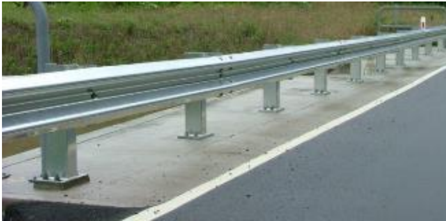
Figure 1: A W-Beam guard rail
