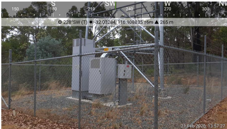
Plate 15: Tele-communications compound west of Weston Road
