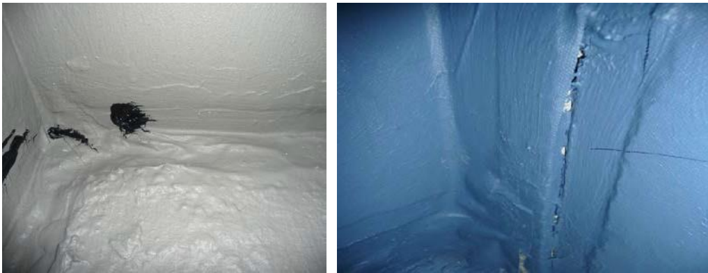
Figure 1 Examples of poorly prepared substrates
