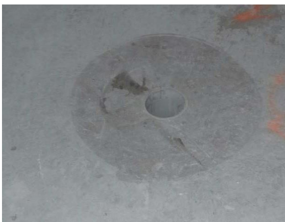
Figure 2 Example of a missing drainage flange
