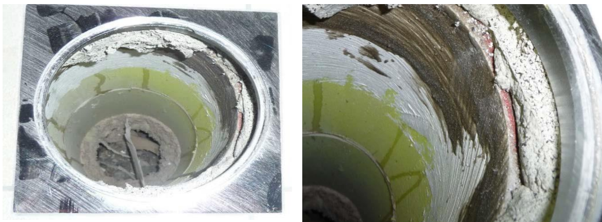
Figure 3 Incorrectly installed membrane at drainage flange
