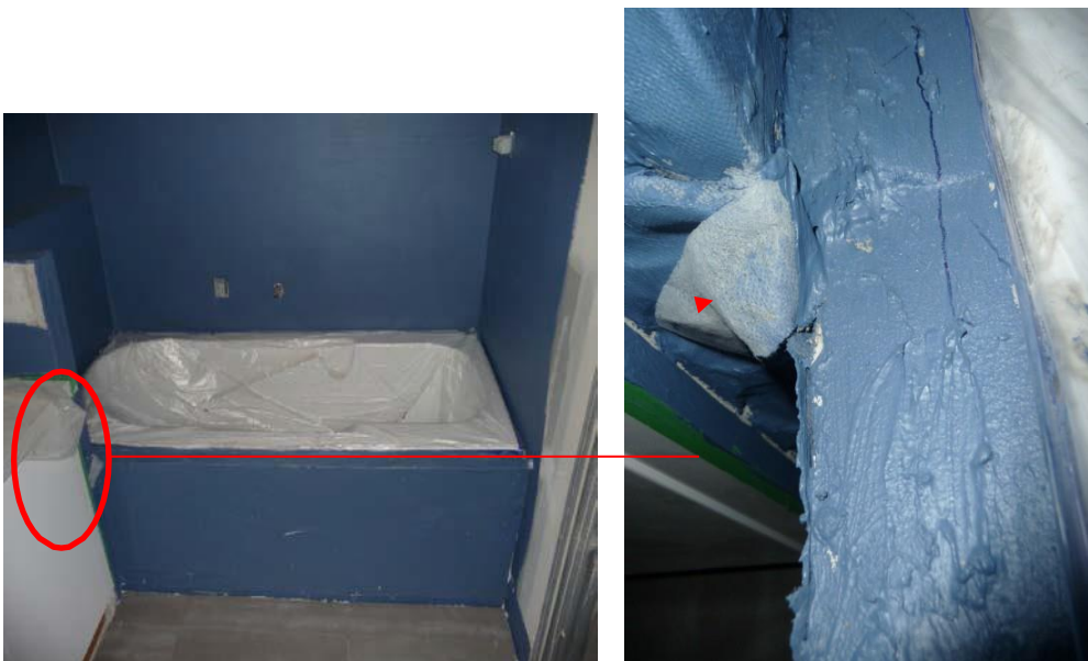
Figure 5 Example of poor workmanship around a bath
