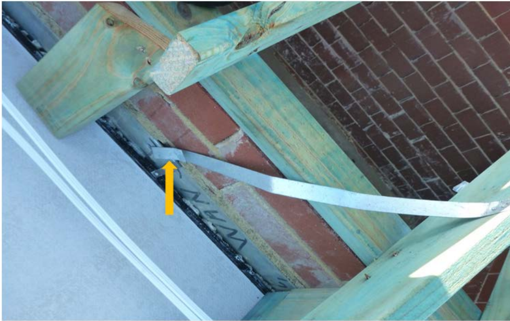
Figure 11. Photograph showing tie-down strap looped through a slot in a lintel
