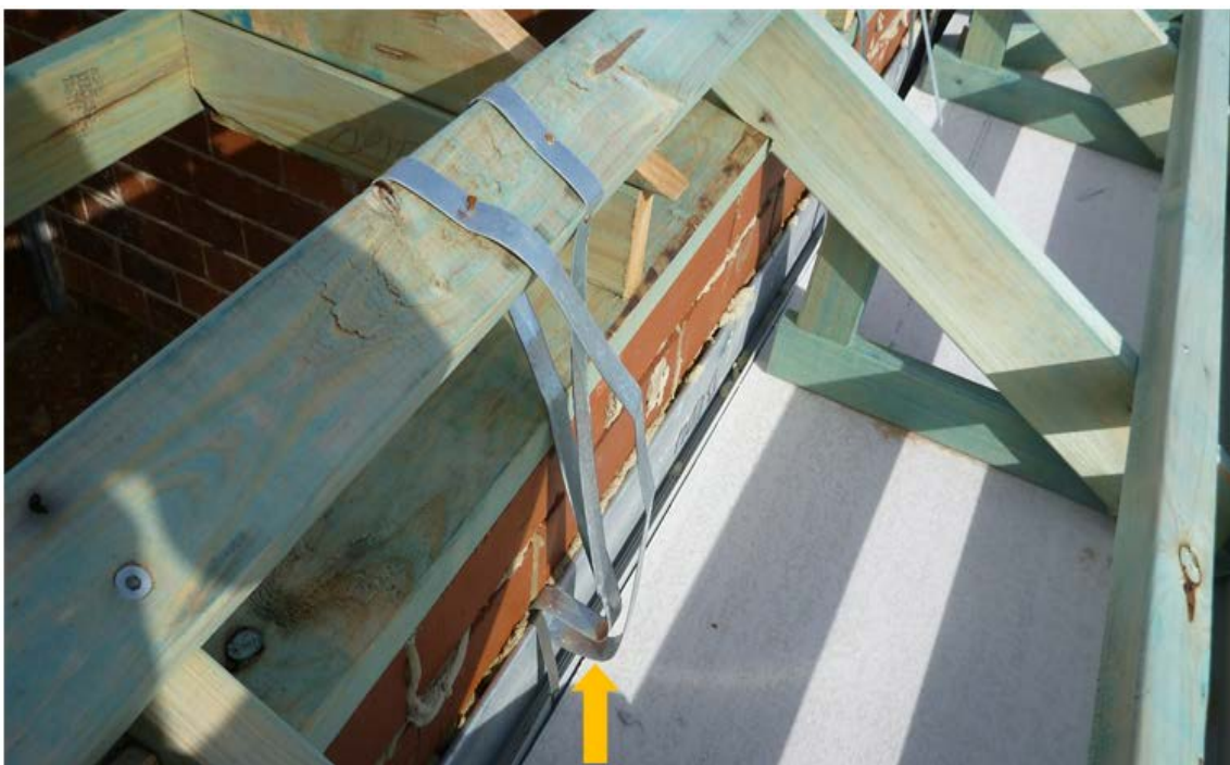
Figure 13. Photograph showing poor installation of tie-down straps
