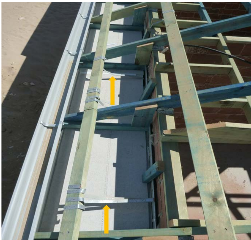
Figure 10. Photograph showing poor tie down strap installation (strap being fixed down the roof line)
