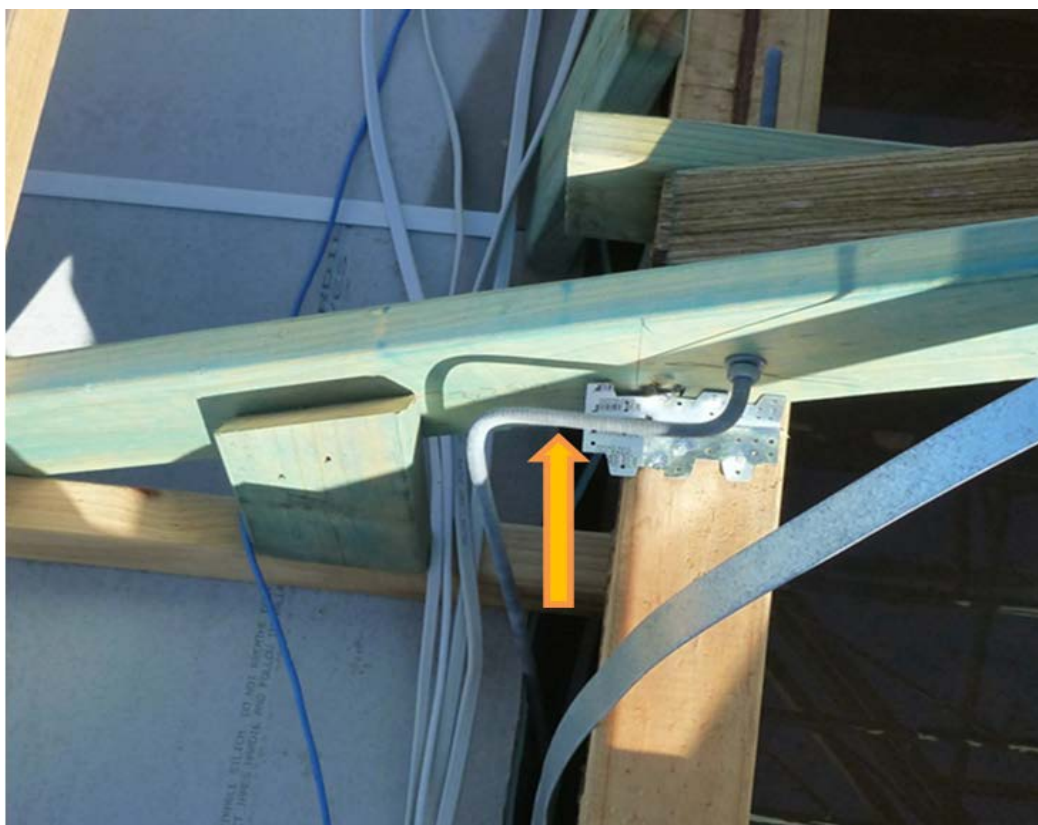
Figure 26. Photograph showing a tie down rod bent to make the connection to the beam
