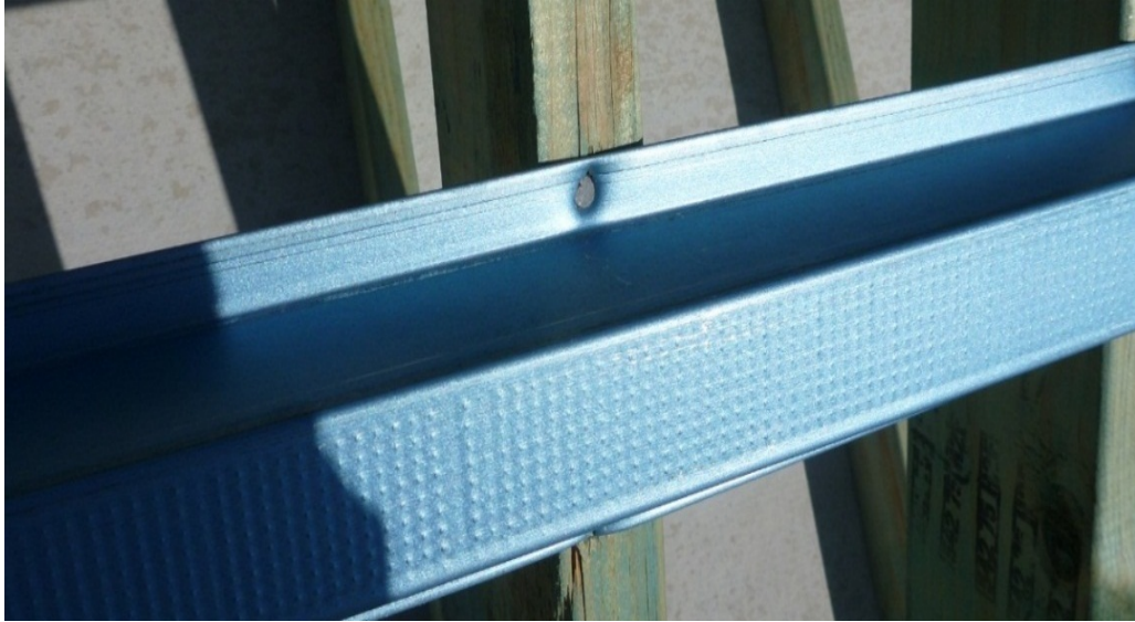
Figure 18. Photograph showing a 75mm x 3.06mm nail over driven when used to fix a metal batten
