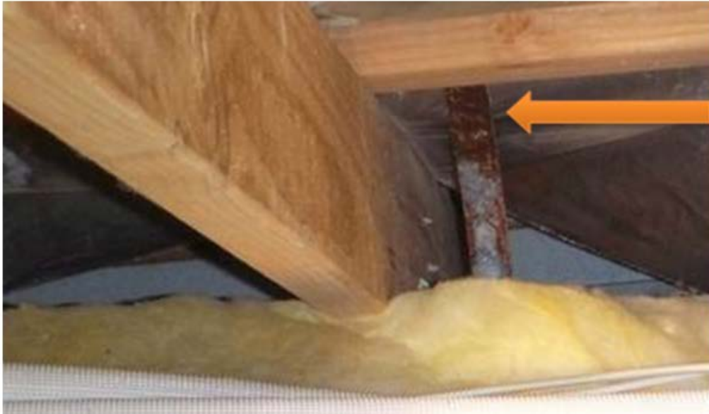
Figure 8. Photograph showing the result of installing a strap without the correct corrosion protection
