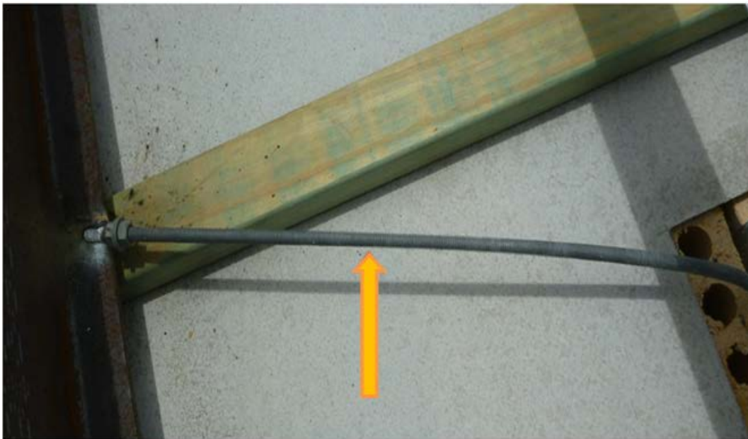
Figure 27. Photograph shows poor installation of a bent tie down rod
