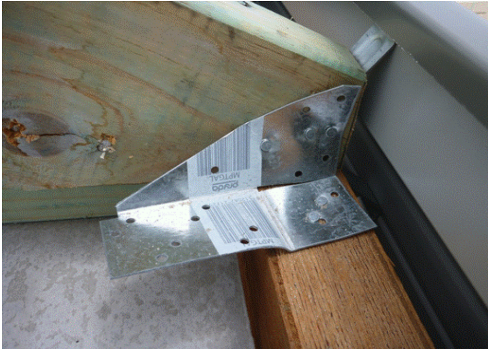
Figure 20. Photograph showing a poorly installed metal connector making the connection between an alfresco beam and rafter
