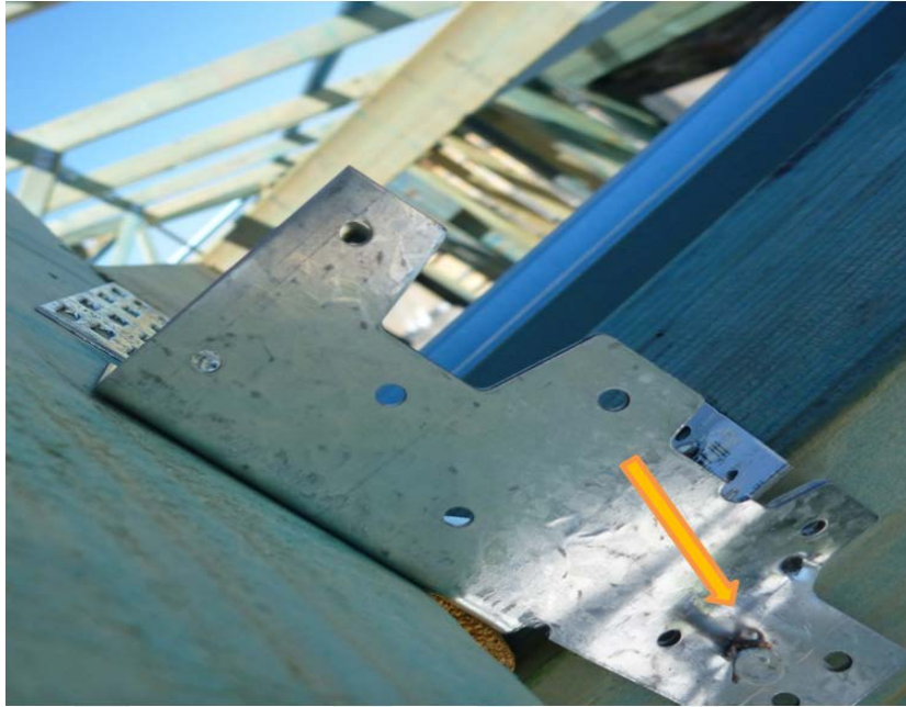
Figure 25. Rafter top plate connection with only one horizontal nail into the top plate tab (Manufacturer recommends 4 nails)
