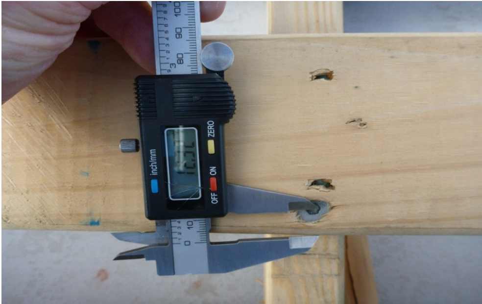
Figure 15. Photograph showing a batten non-compliant screw close to the edge of the batten
