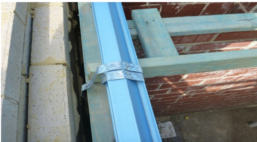
Figure 12. Photograph showing tie-down wrapped around metal batten (Note: the tie down is loose)
