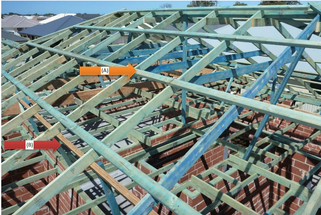
Figure 23. Photograph showing non-compliant collar tie installation
