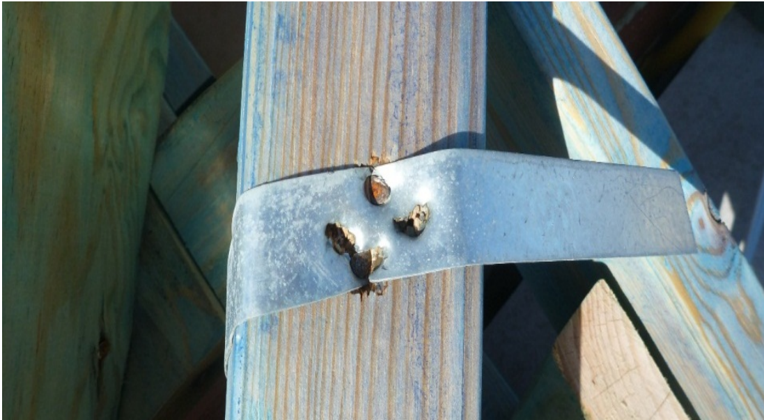
Figure 9. Photograph showing a metal tie-down strap fixed to a batten via the use of machine driven nails. The over-driving of nails has damaged the strap, greatly reducing the connection capacity.
