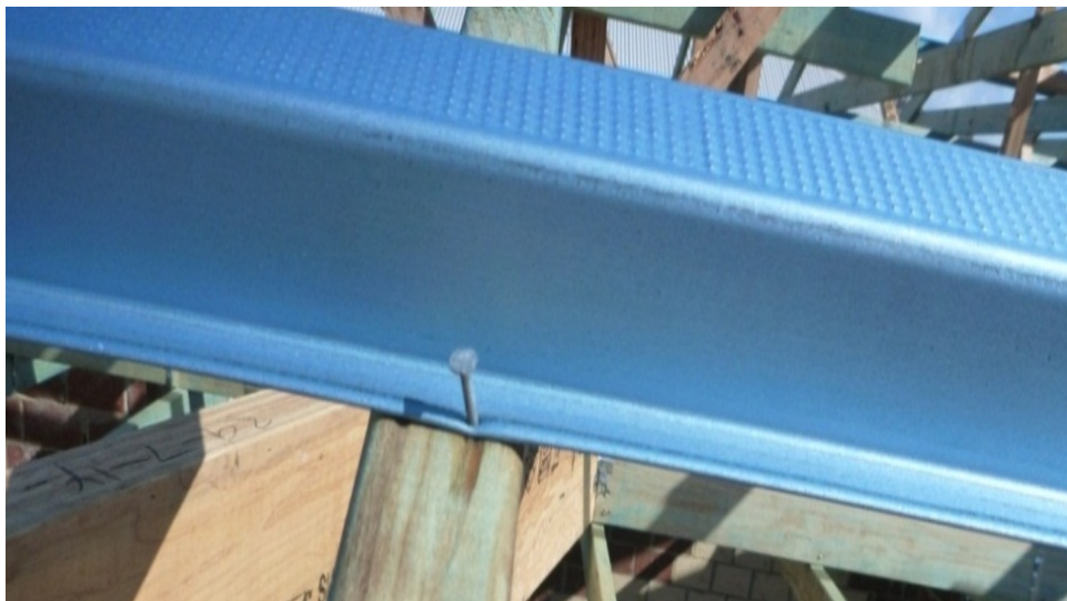
Figure 19. Photograph showing a typical under driven nail fixing a metal batten around this roof
