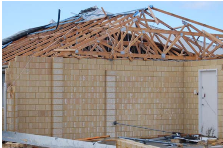
(a) roof batten loss
