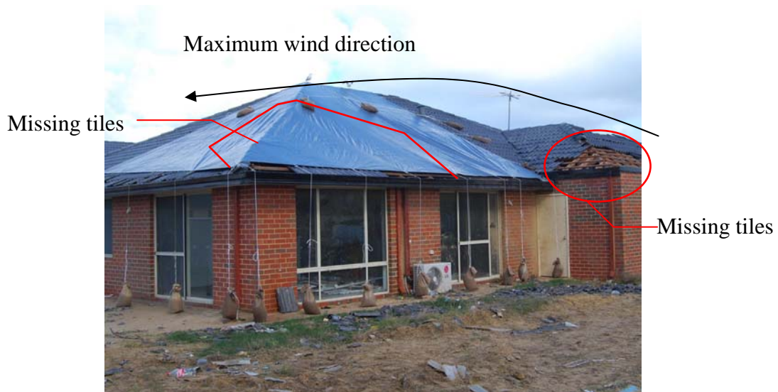
Figure 3.2 Damage to tiled roof due to wind loads
