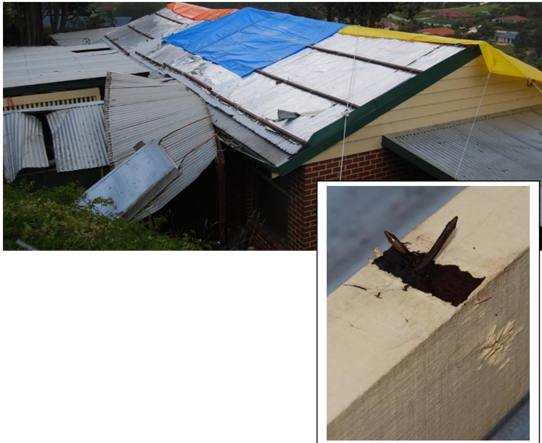
Figure 4.10 Batten loss from older truss roof (inset shows small depth of penetration of nails in softwood trusses)
