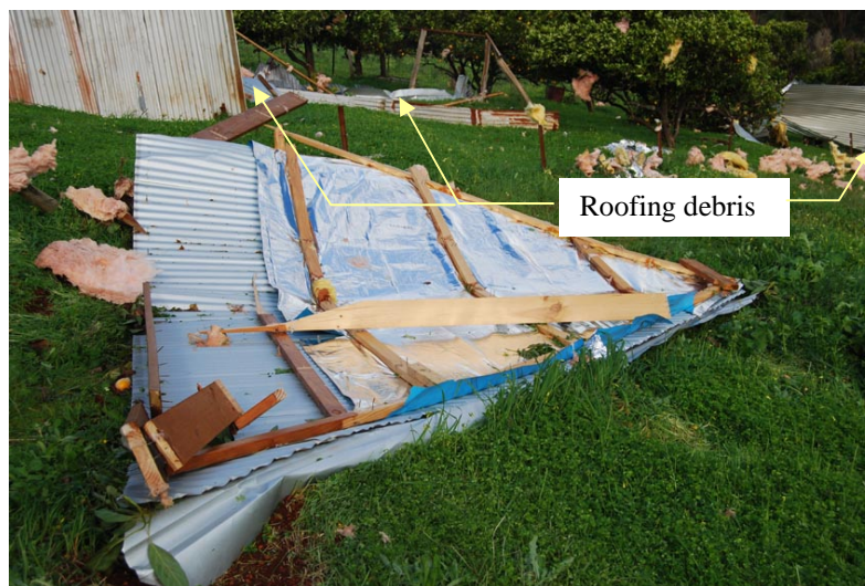
Figure 4.14 Debris strewn more than 50 metres from house
