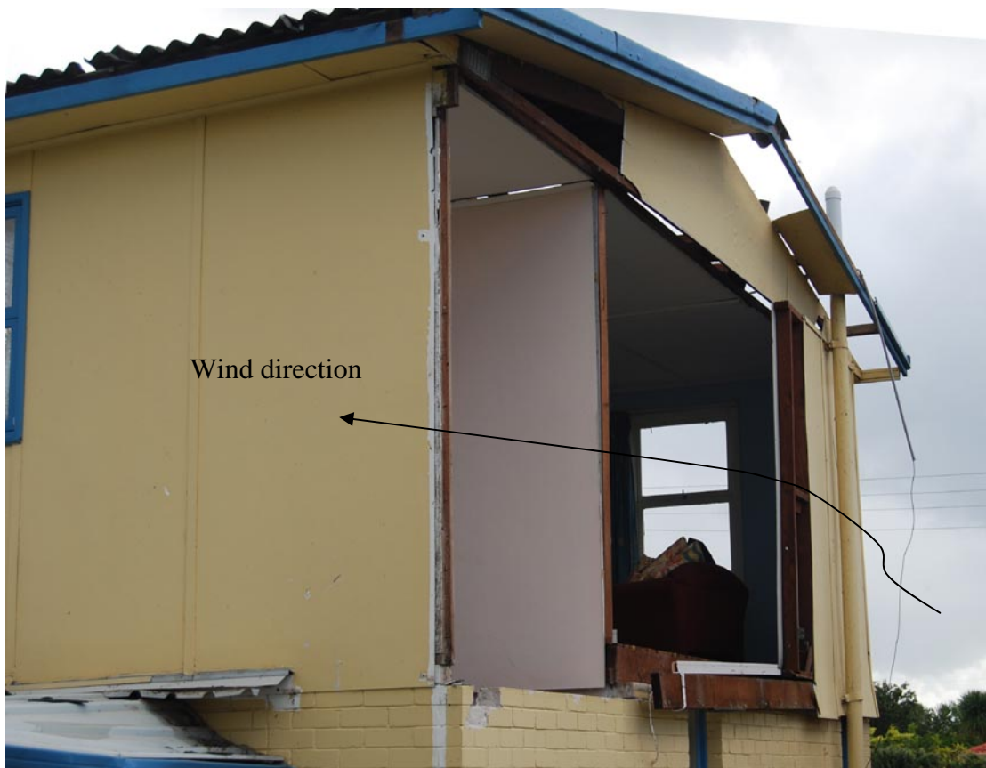
Figure 4.12 Loss of a side wall under combined internal pressure and external suction
