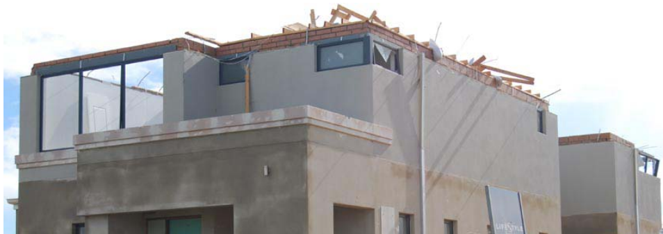
(a) Upper storey with loss of most of roof structure
