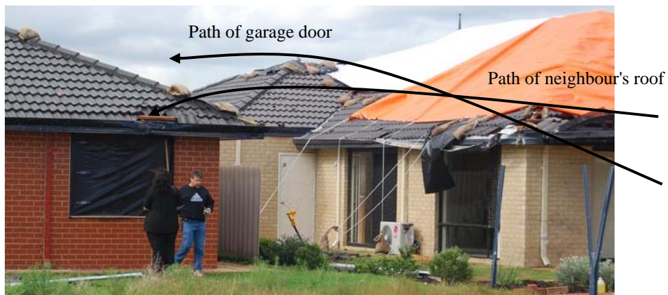
Figure 4.13 Debris damage to tiled roofs
