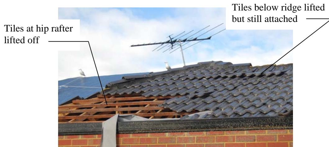
Figure 4.2 tiles in high uplift regions of the roof.
