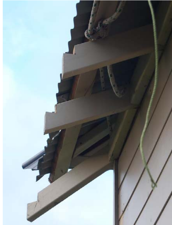
(b) lifted roof battens near corner of roof
