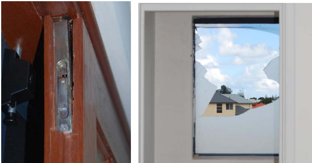
(a) broken door furniture
