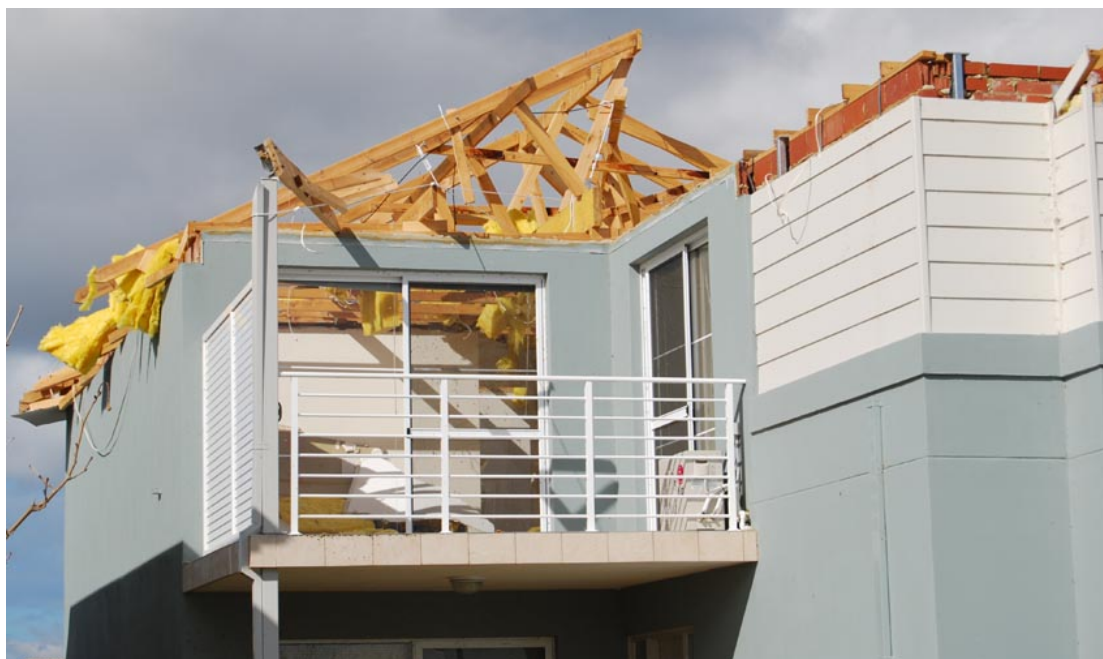
Figure 4.7 Loss of roof structure – two storey house
