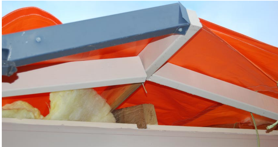
(a) failure of truss anchorage
