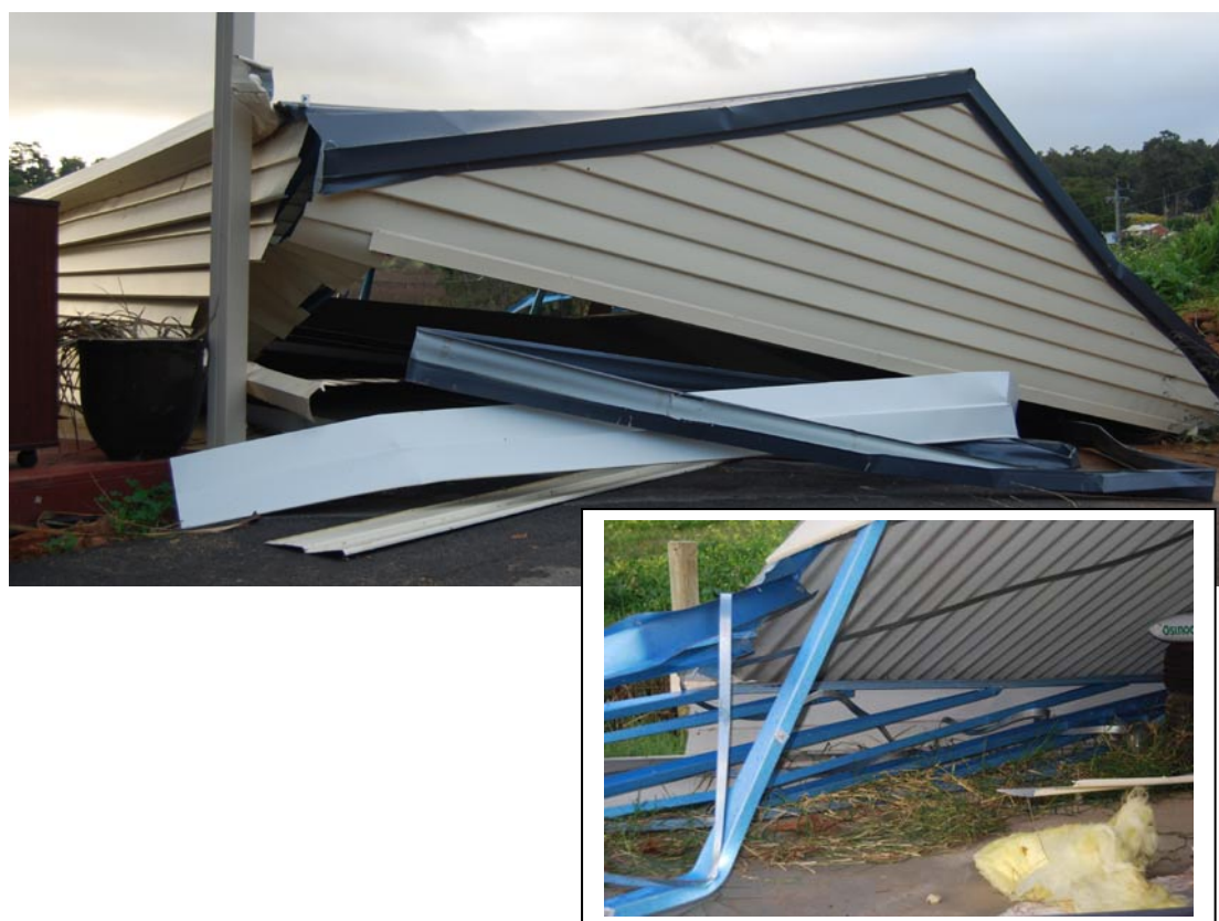
Figure 4.15 Racking failure of garage
