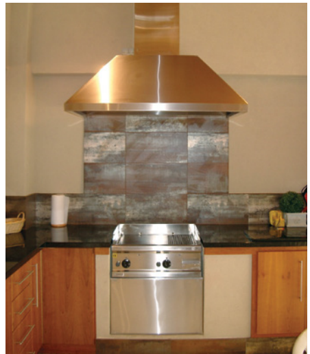
A commercial gas barbecue with mechanical ventilation.
