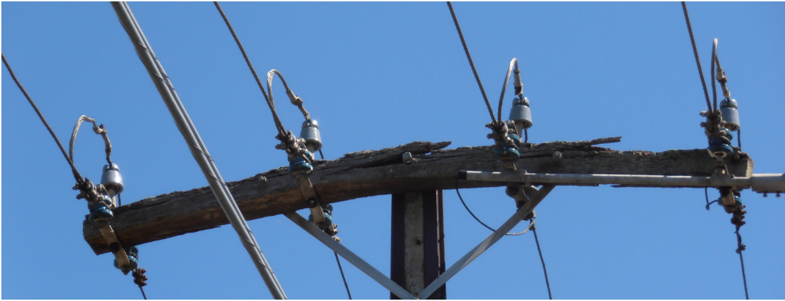
FIGURE 8 – A BADLY SPLIT LOW VOLTAGE CROSSARM
