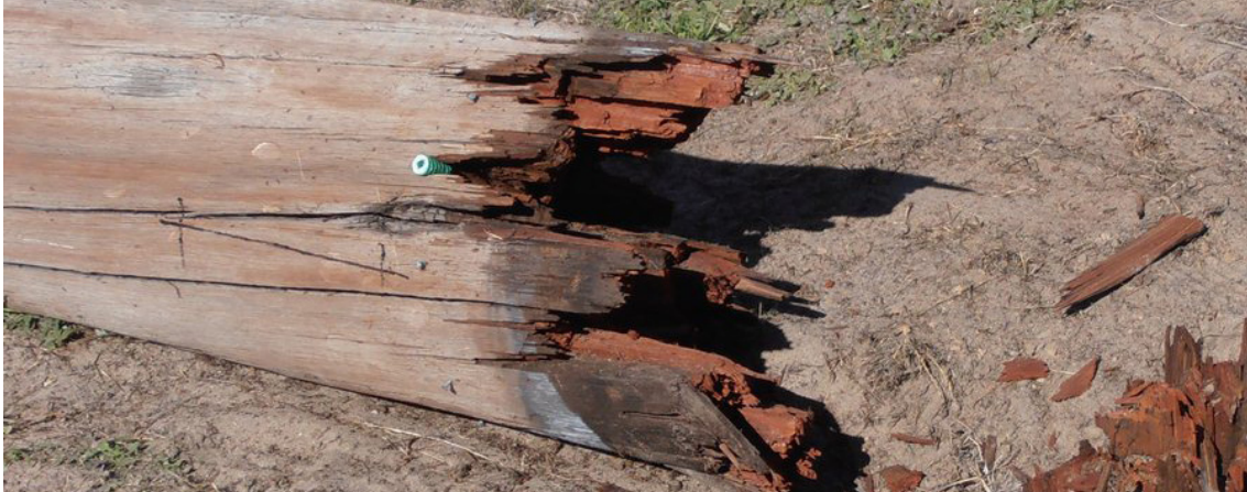
FIGURE 6 – COMPLETE FAILURE OF JARRAH WOOD POLE DUE TO DECAY/ROTTING
