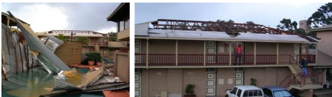
(a) Damage to a two-storey commercial property in 2004. The original tiled roof was replaced with a metal sheeted roof.
