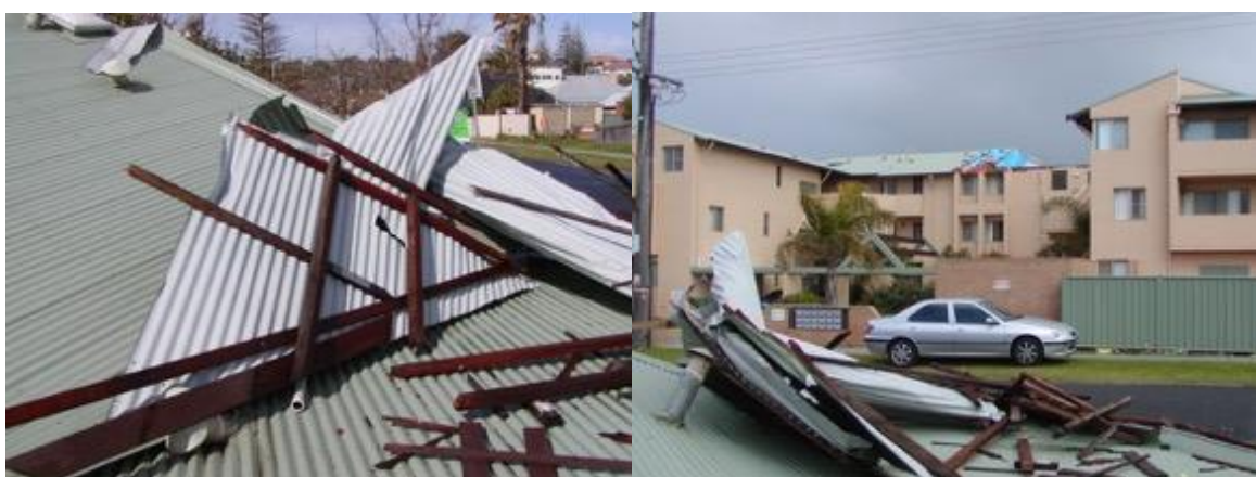
(b) Damage to an apartment building during a storm in 2004. The original tile roof was replaced with metal sheet roof. The roof cladding and part of the roof structure damaged a neighbouring building.
