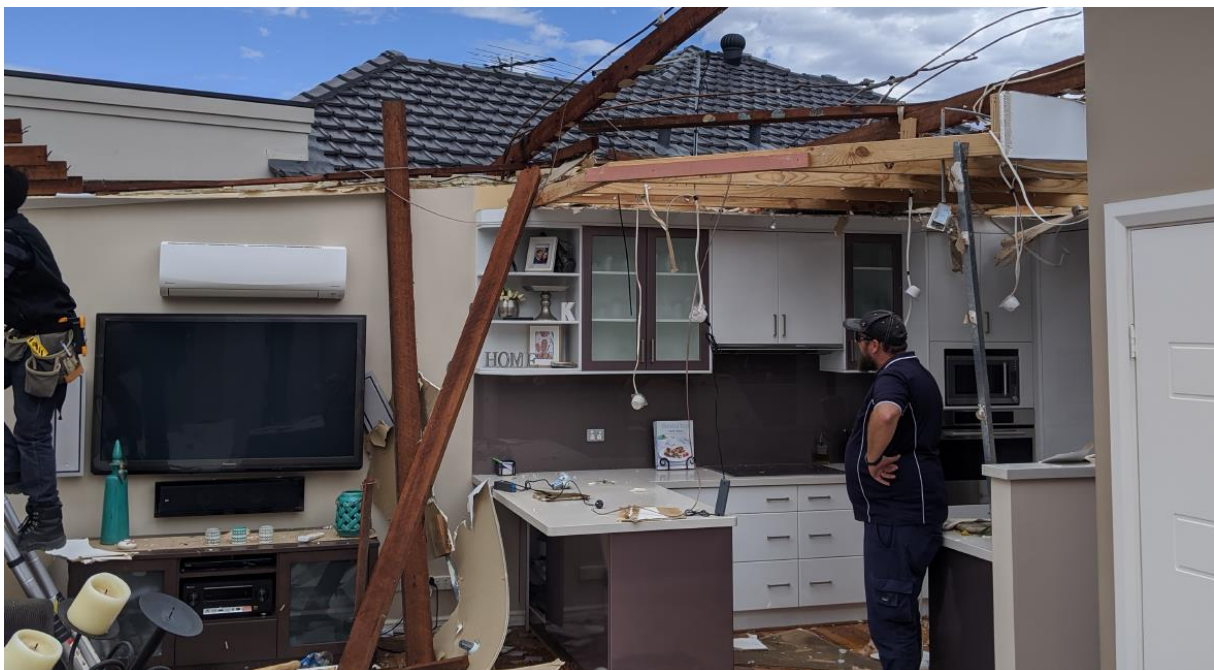
(e) Damage to a two-storey house built in 1979. The original asbestos roof sheeting was replaced with a metal sheet roof in 2004. The roof was lost during a storm in February 2020 with the owners still awaiting completion of repair works prior to moving back into their home at the time of this report
