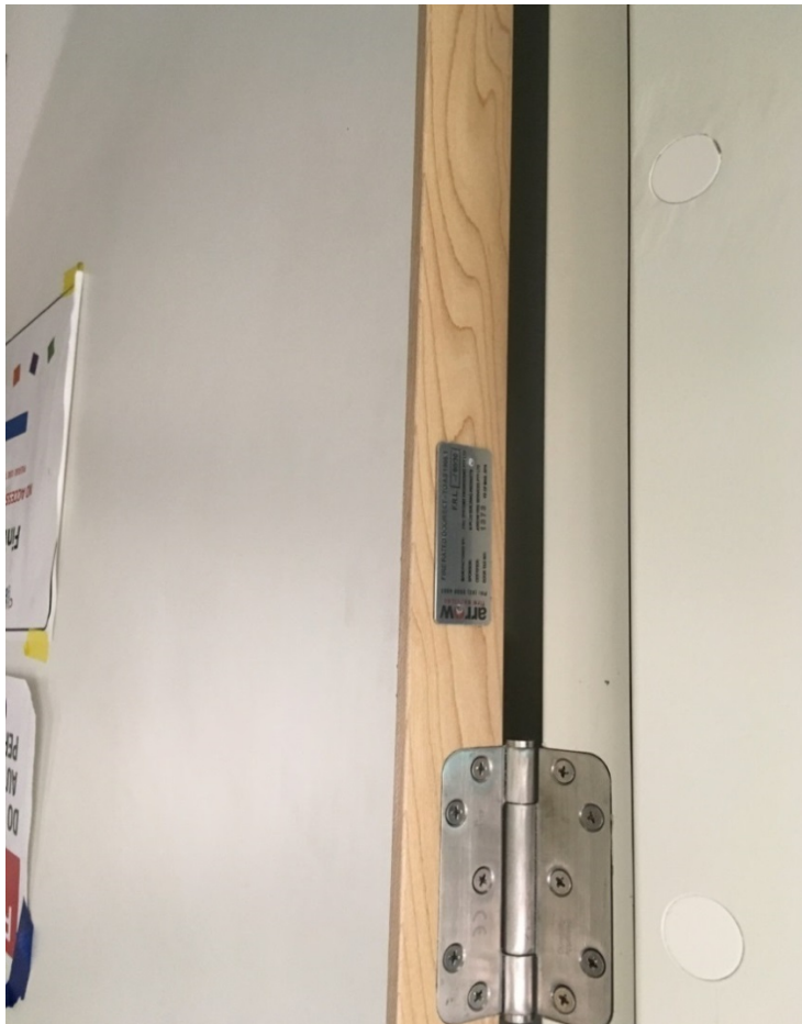
Photograph 12: Fire rated doorset
