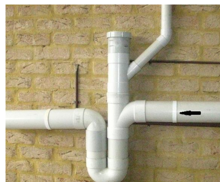
Photo 1: Sealed and vented trade waste sampling point
