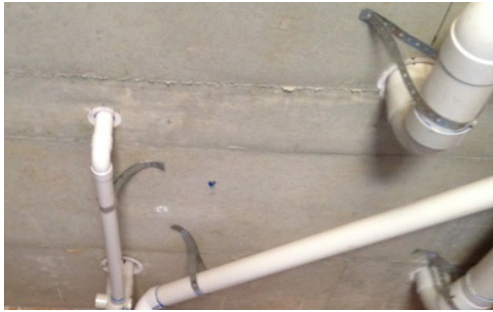
Photo 8: Non-compliant fabricated hoop iron clips on sanitary pipework
