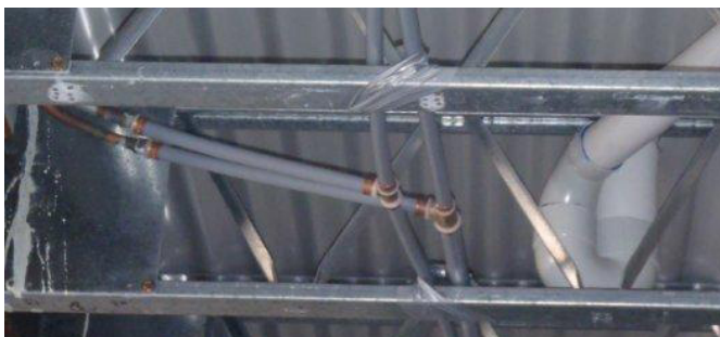
Photo 1: Non-compliant clipping using duct tape.
