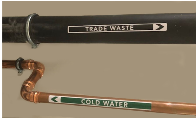
Photo 11: Compliant labeling of pipework
