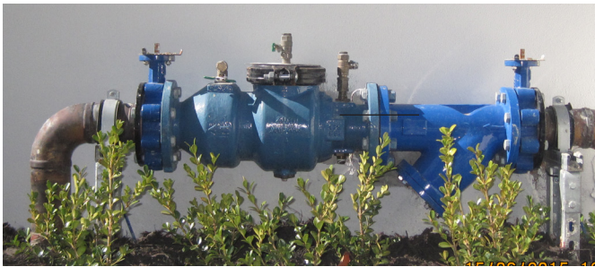
Photo 5: Compliant support of external valves.
