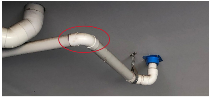
Photo 9: Non-compliant bend support of sanitary pipework as per AS/NZS 2032
