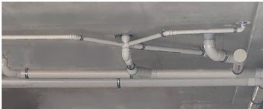
Photo 10: Compliant clipping at all bends in sanitary pipework in accordance with AS/NZS 2032
