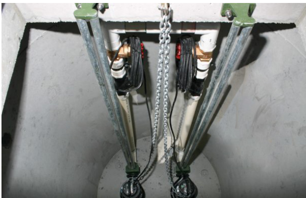
Photo 1: Typical wet well installation
