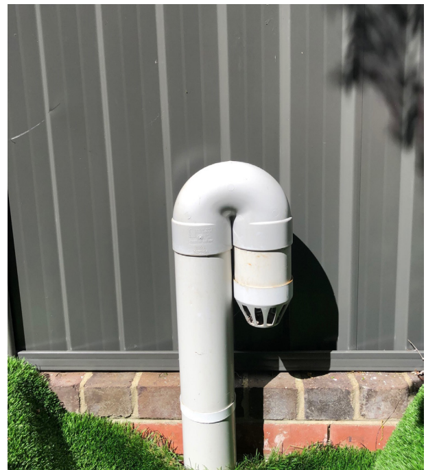
Photo 2: Example of low level vent termination
