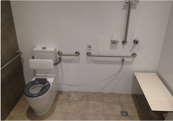
Photo 2: Non-compliant facility with shower head below rim of the toilet pan
