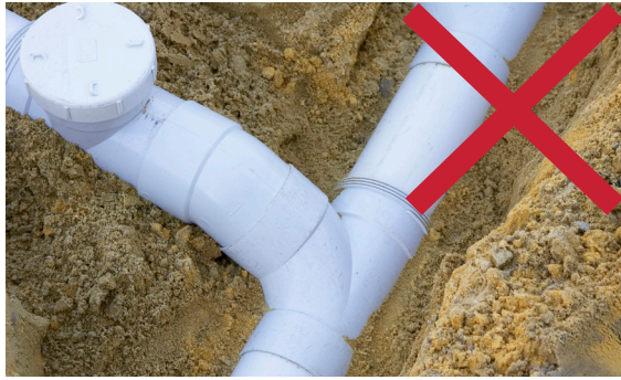
Photo 1: 88° junctions not permitted on graded drains
