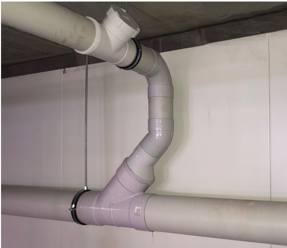
Photo 4: 45° junction on back forming a vertical riser
