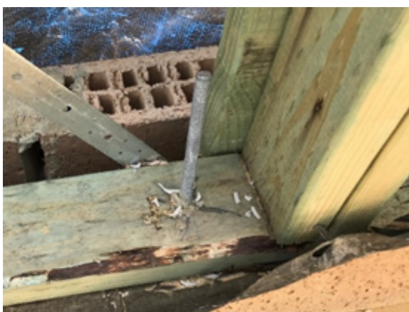
Figure 2 above. No nut or washer installed to holding down bolt as required by approved engineering plans.
