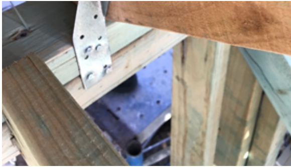
Figure 1, inappropriate number of machine driven nails used with insufficient spacings to existing holes.
