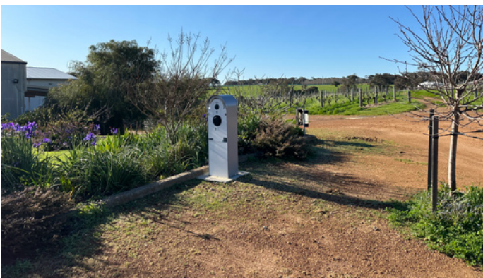
Image of one of Juniper's EV chargers installed at its cellar door in Cowaramup. Supplied by Juniper, September 2024.
