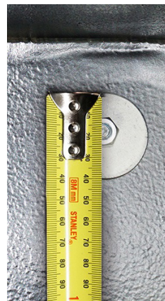
Clearly show the size of the washers by using a ruler for scale
